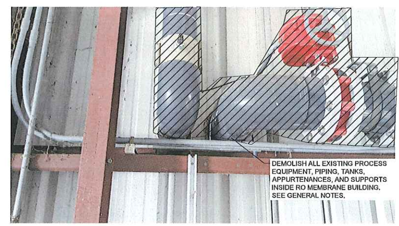
TT PHOTO FILE: RO FILTRATION BUILDING INTERIOR-4-4
