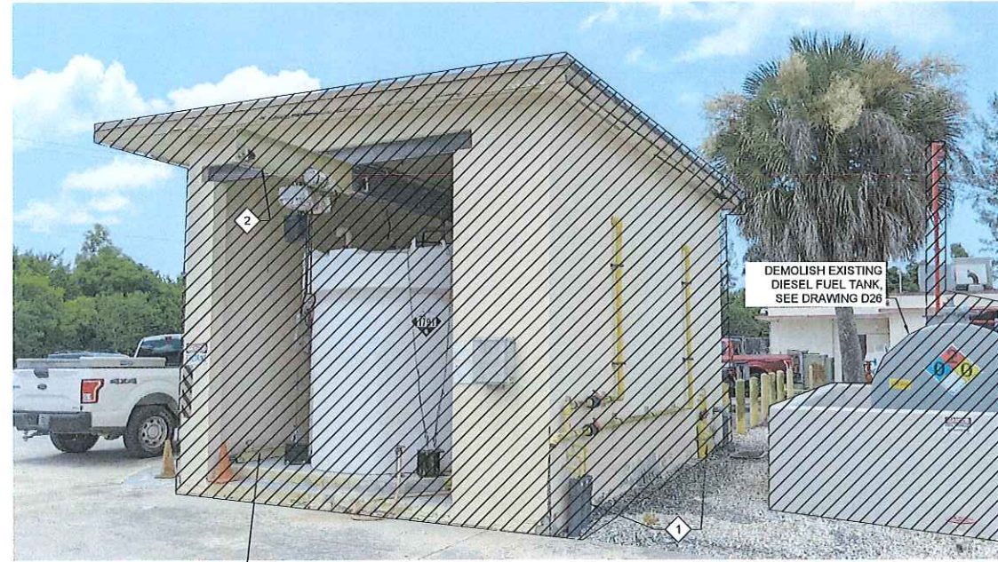
DEMOLISH AND DISPOSE OF CHLORINE STORAGE BUILDING AND ITS CONTENTS IN ENTIRETY, SEE GENERAL NOTES
