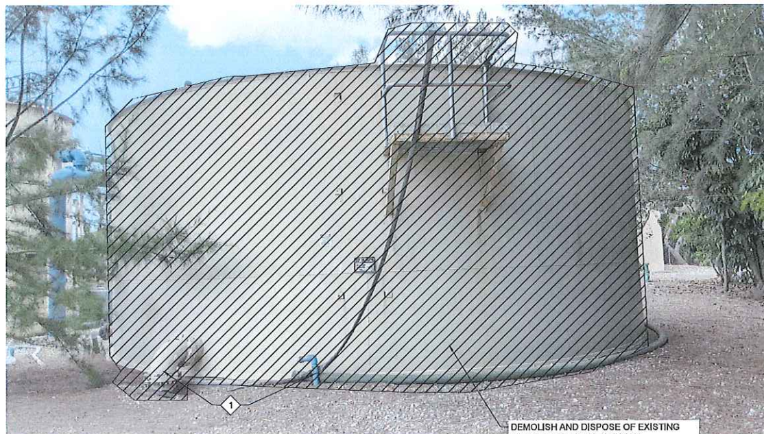
BG PHOTO FILE: FILTER BAKWASH TANK -2
