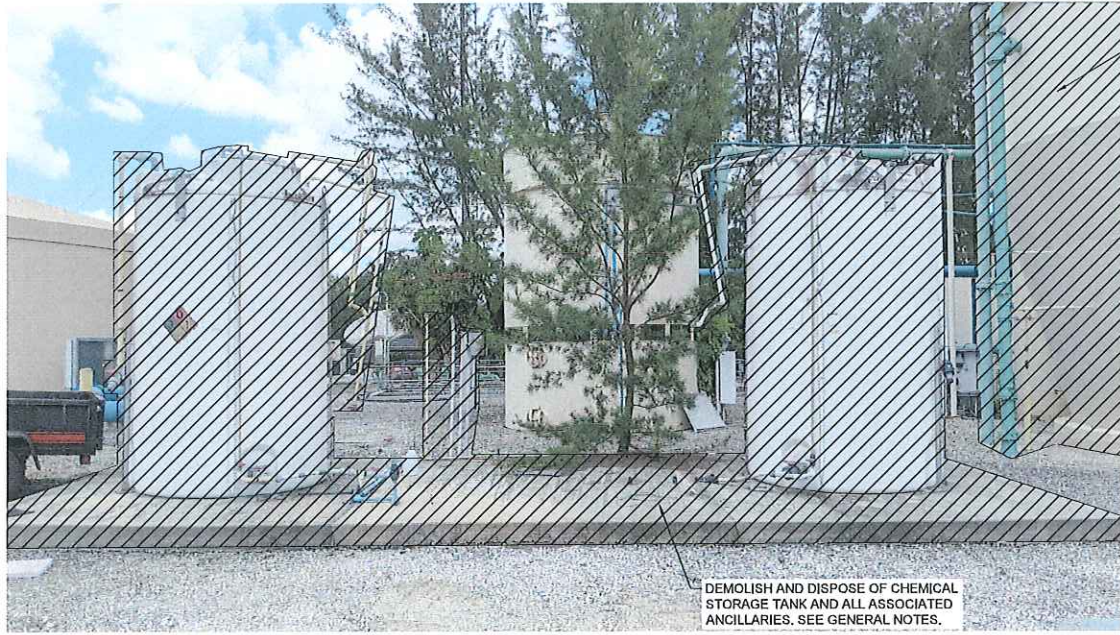
AN PHOTO FILE: CHEMICAL STORAGE TANK-1
