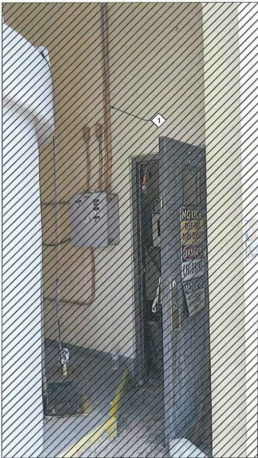
CC PHOTO FILE: CHLORINE STORAGE BUILDING 2-5
