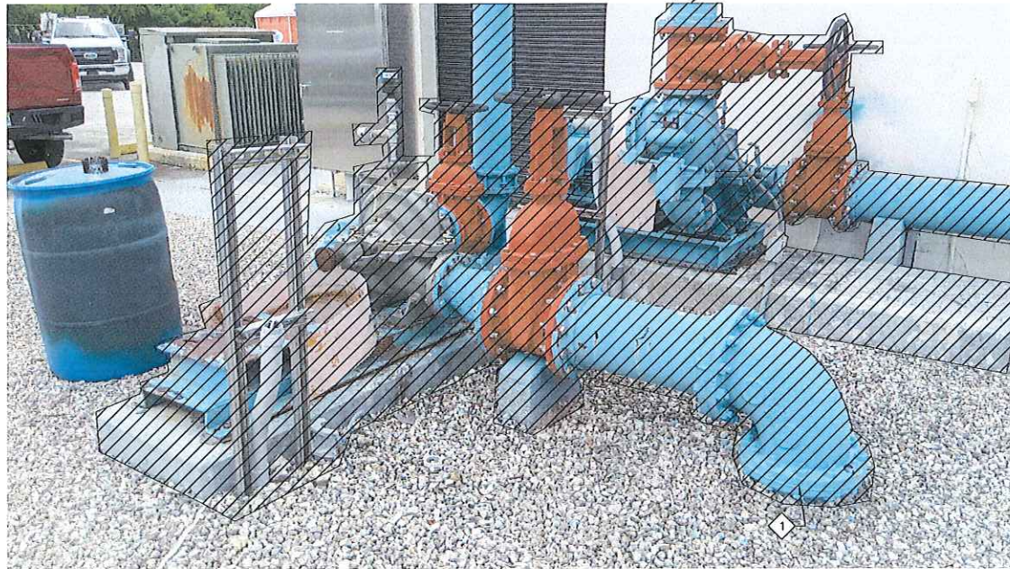
CK PHOTO FILE: HIGH SERVICE PUMP #3-3
