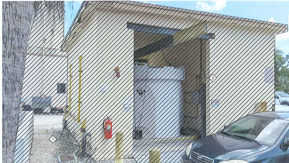
DEMOLISH AND DISPOSE OF CHLORINE STORAGE BUILDING AND ITS CONTENTS IN ENTIRETY, SEE GENERAL NOTES
