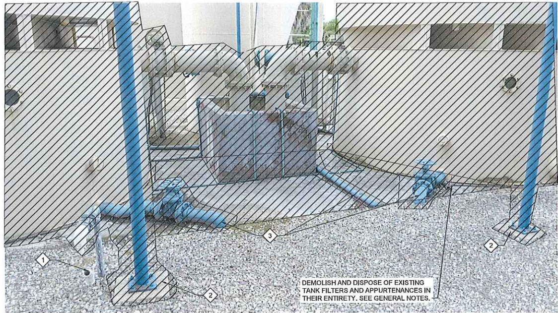
AW PHOTO FILE: TANK FILTERS 2-1
