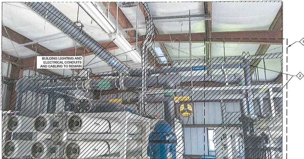
SS PHOTO FILE: RO FILTRATION BUILDING INTERIOR-4-3
