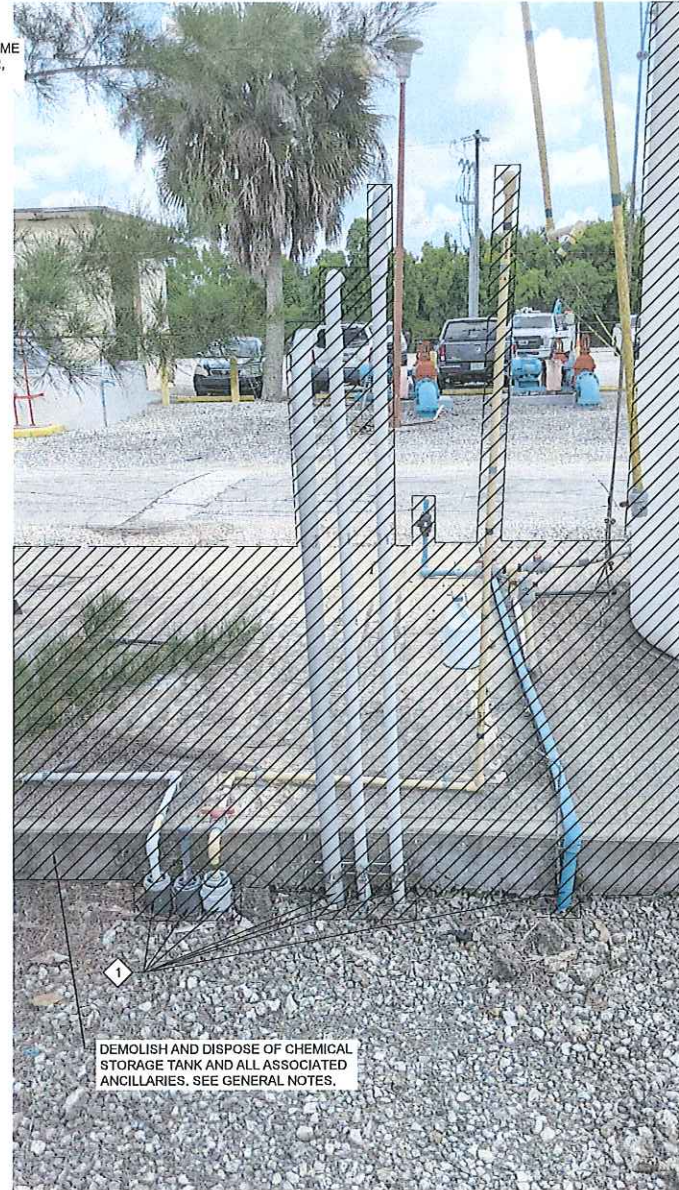
AQ PHOTO FILE: CHEMICAL STORAGE TANK-2
