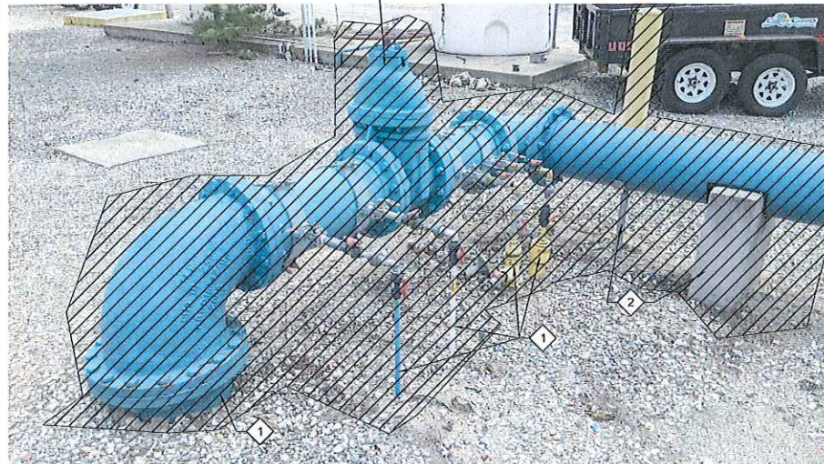
DEMOLISH AND DISPOSE OF ABOVE GRADE INJECTION POINT 2 PIPING AND APPURTENANCES. SEE GENERAL NOTES.
