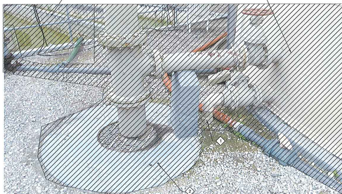
BI PHOTO FILE: FILTER BAKWASH TANK -4
