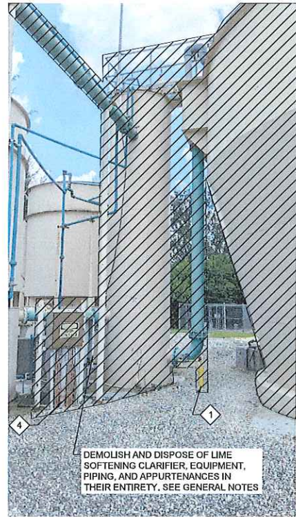
AL PHOTO FILE: LIME SOFTENING CLARIFIER-7
