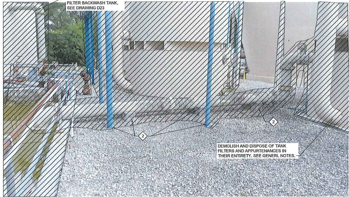
AX PHOTO FILE: TANK FILTERS 2-2
