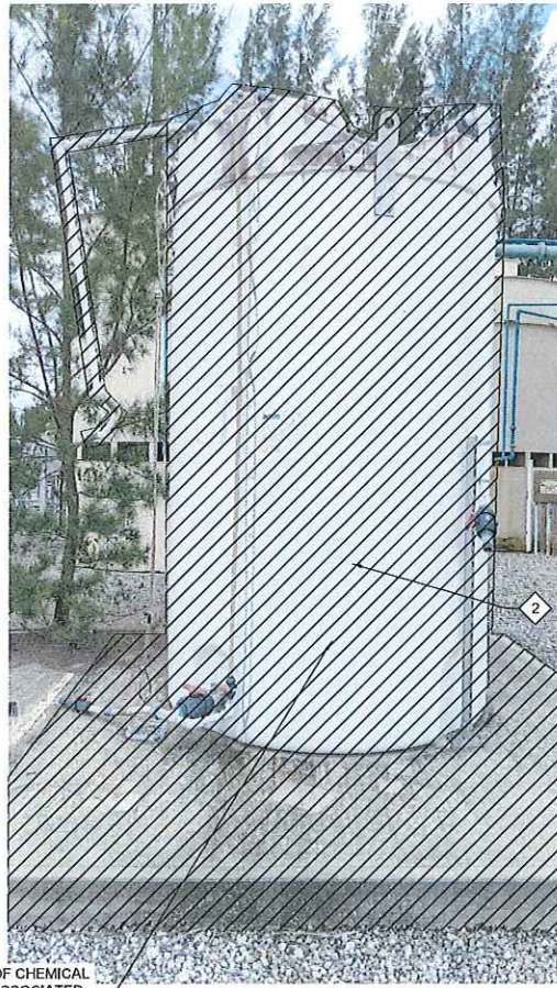
AP PHOTO FILE: CHEMICAL STORAGE TANK-4
