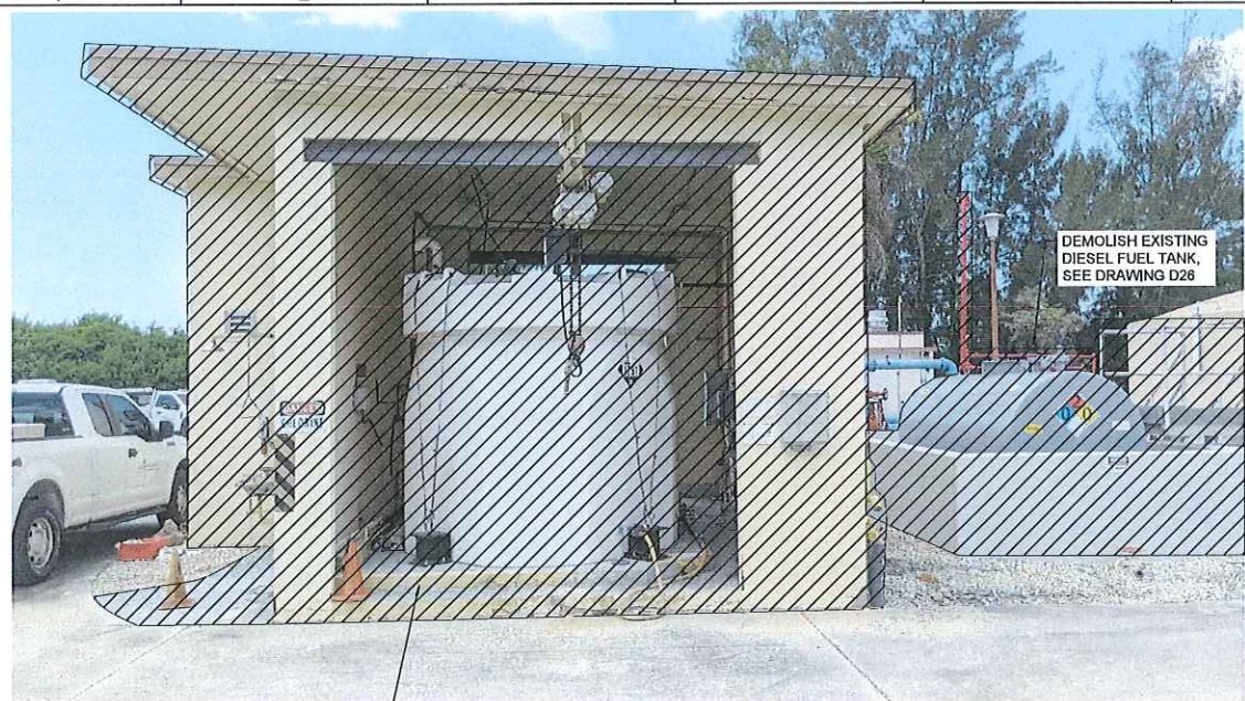
DEMOLISH AND DISPOSE OF CHLORINE STORAGE BUILDING AND ITS CONTENTS IN ENTIRETY. SEE GENERAL NOTES.
