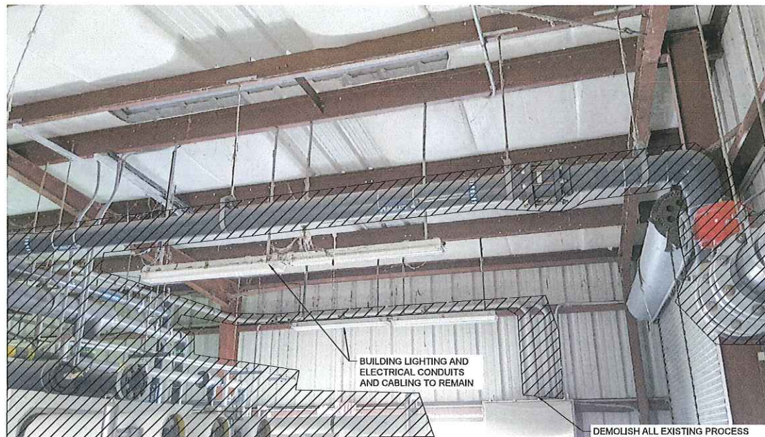
RR PHOTO FILE: RO FILTRATION BUILDING INTERIOR-4-2
