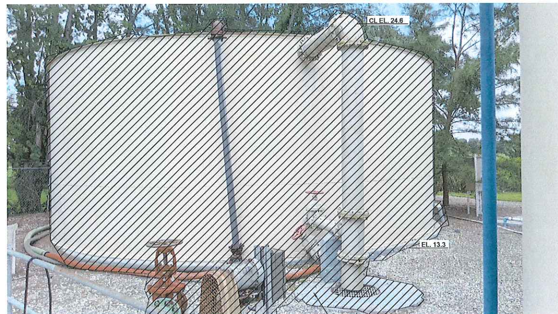
BF PHOTO FILE: FILTER BAKWASH TANK -1
