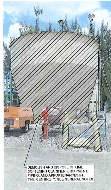
AF PHOTO FILE: LIME SOFTENING CLARIFIER-1
