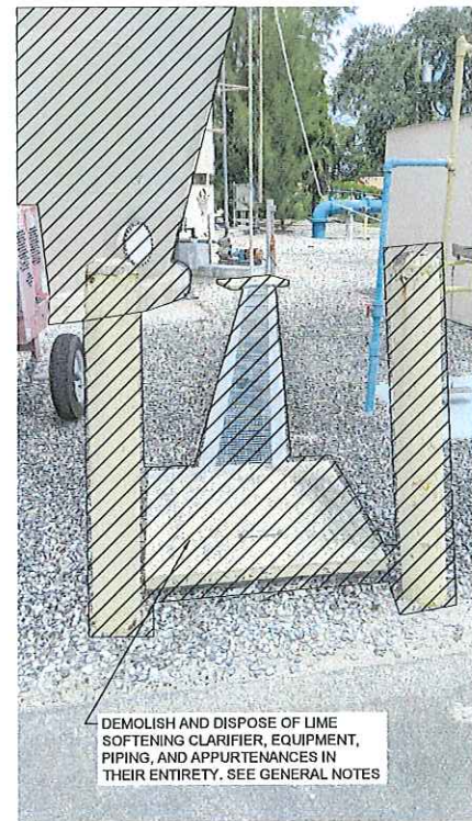
AJ PHOTO FILE: LIME SOFTENING CLARIFIER-5
